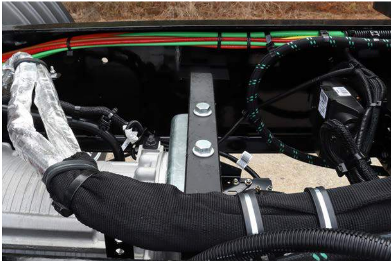
FMM COOLANT LINE INSULATION coolant lines are insulated as part of the prep for the CNG System
